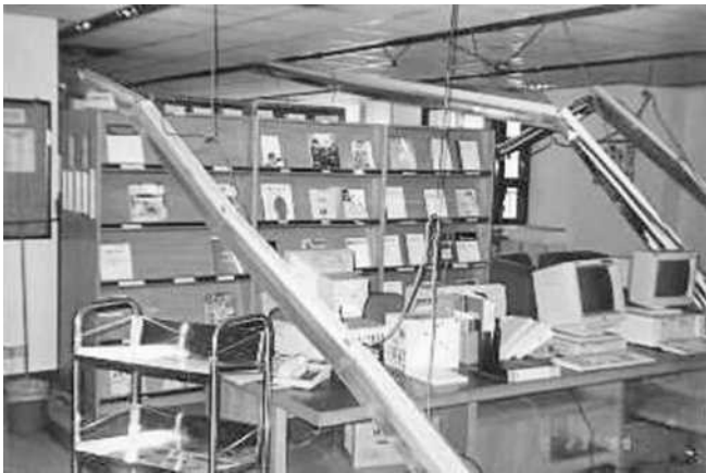
FIGURE C13.1-3 Collapsed Light Fixtures
