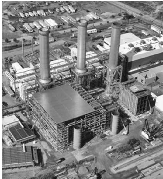
FIGURE C15.1-3 Heat recovery steam generators
