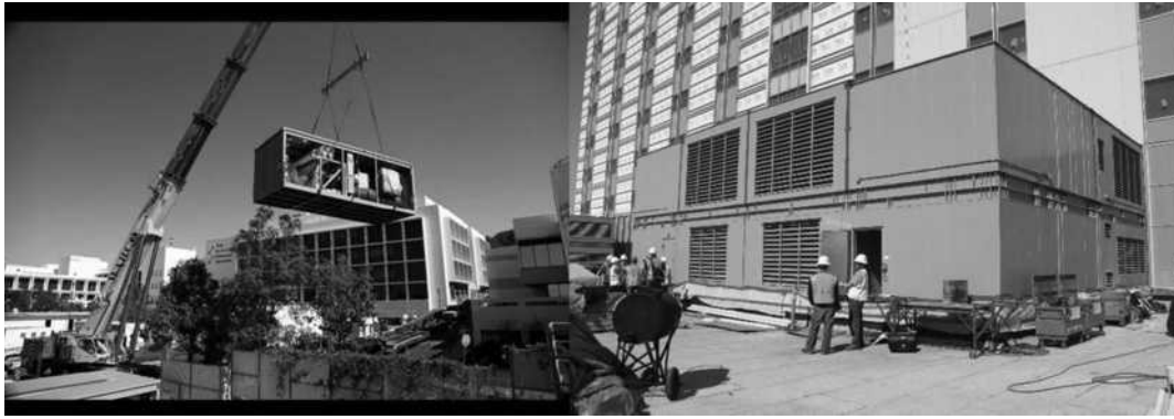
FIGURE C13.1-7 Premanufactured Modular Mechanical Systems
