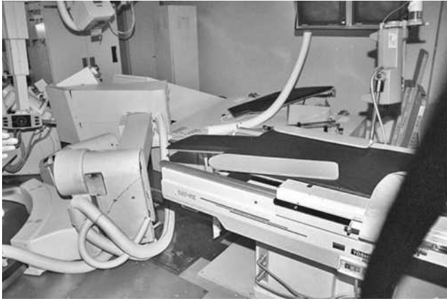
FIGURE C13.1-1. Hospital Imaging Equipment That Fell from Overhead Mounts
