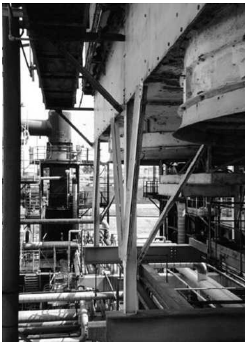
FIGURE C13.6-1 Fin Fan Elevated on Integral Supports
